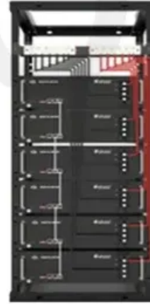
Cabinet and rack installation display
